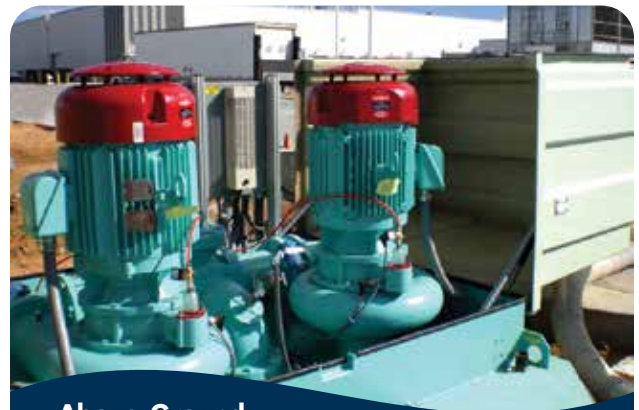
Above-Ground Duplex Pump Station for Process Wastewater
