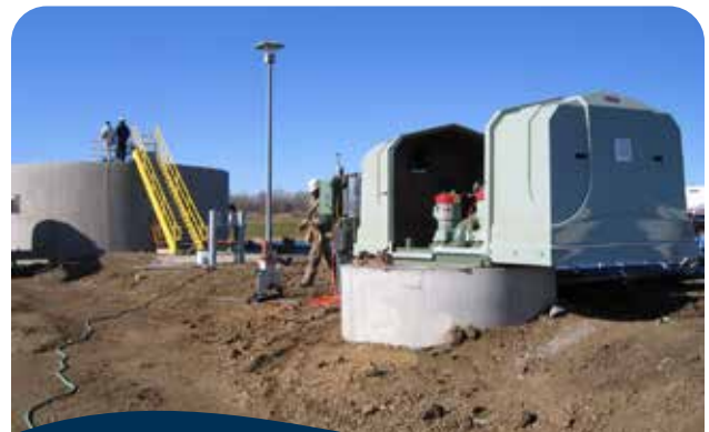
Above-Ground Duplex Pump Station for Process Wastewater
