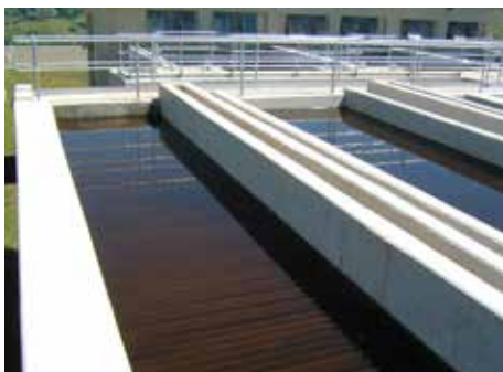
Upgrade from large settling tanks that can require higher chemical use to enhance settling and large volumes of facility space.
