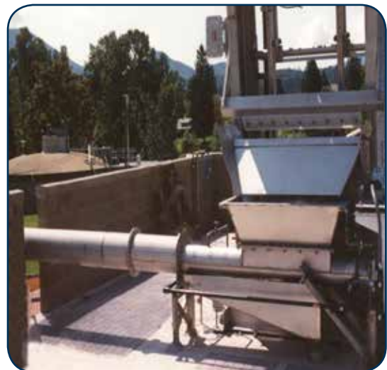
Screenings conveyor, washer and compactor
