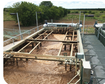
S&L MBR Tank [factory-built with membranes]
